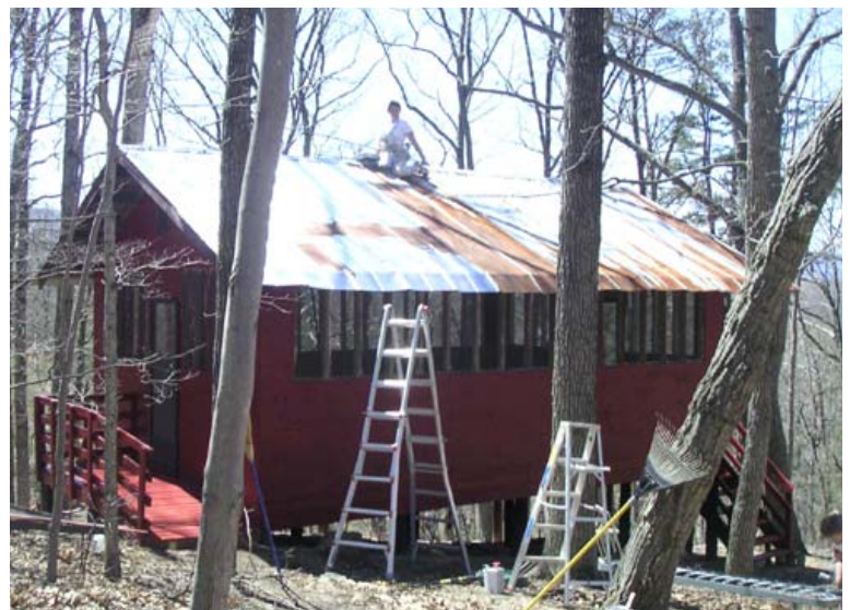
Above: PROM Committee Chairman, Amy Tubbs, helps rust coat the cabins during the April work weekend.
